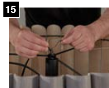
15 Loop same end of aircraft cable through balancer.
